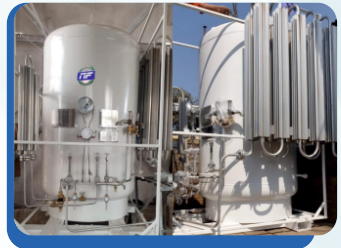
01KL CRYOGENIC STORAGE TANK
